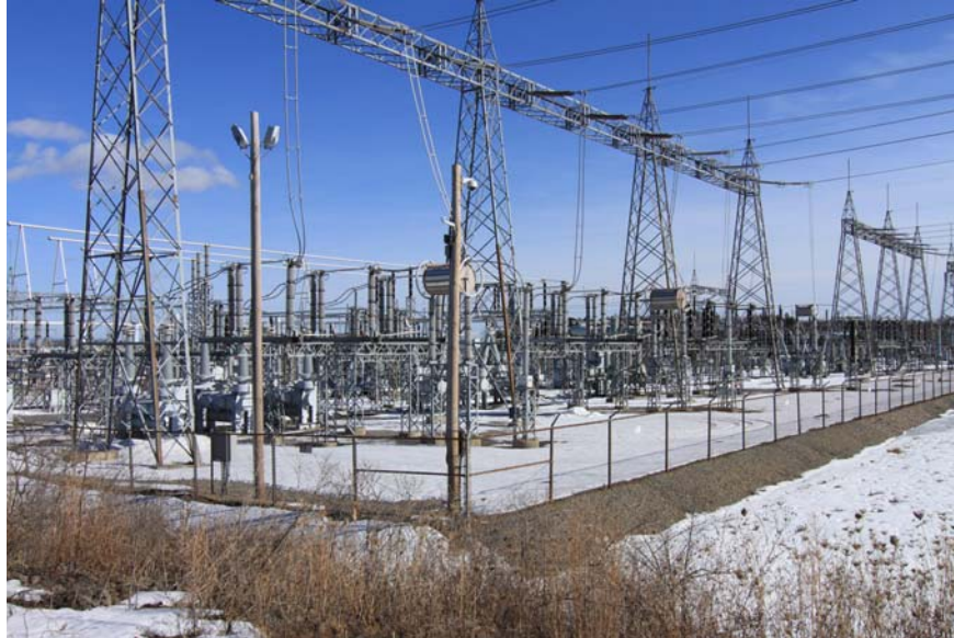
Figure 5 Critical components of the electric grid can be secured with wireless detectors connected to PTZ cameras
