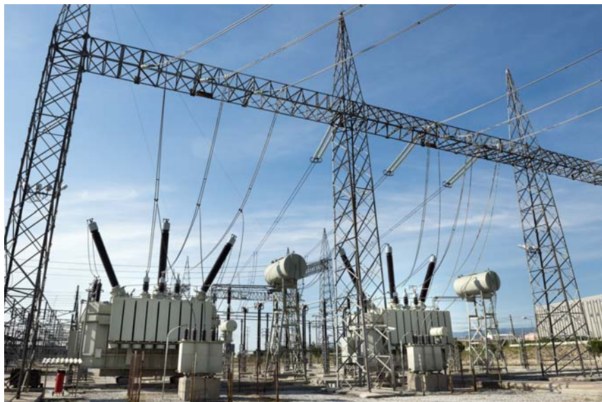
Figure 3 The transformers that make up the electrical grid are easily disabled with only a basic knowledge of their design
